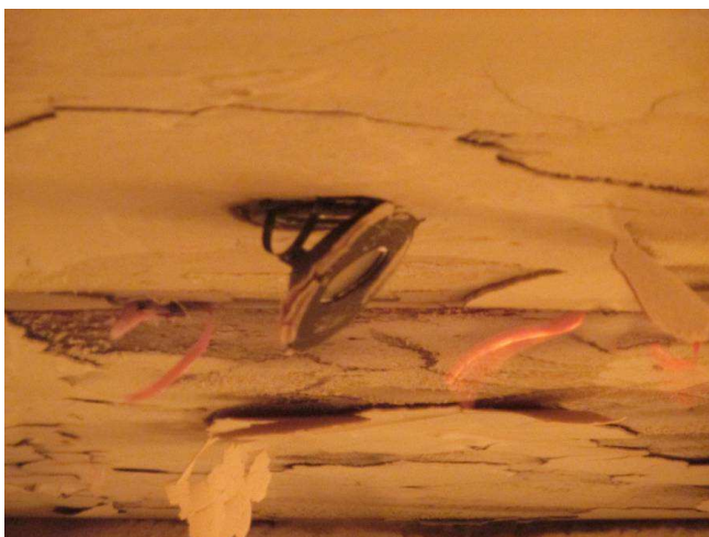
Photo 15: The exposed surface of the specimen after test duration of 16 minutes, showing the faceplate of specimen was falling away.
