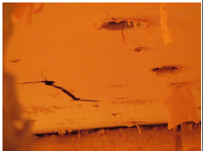
Photo 16: The exposed surface of the specimen after test duration of 28 minutes, showing some cracks appeared on the first layer plasterboard ceiling
